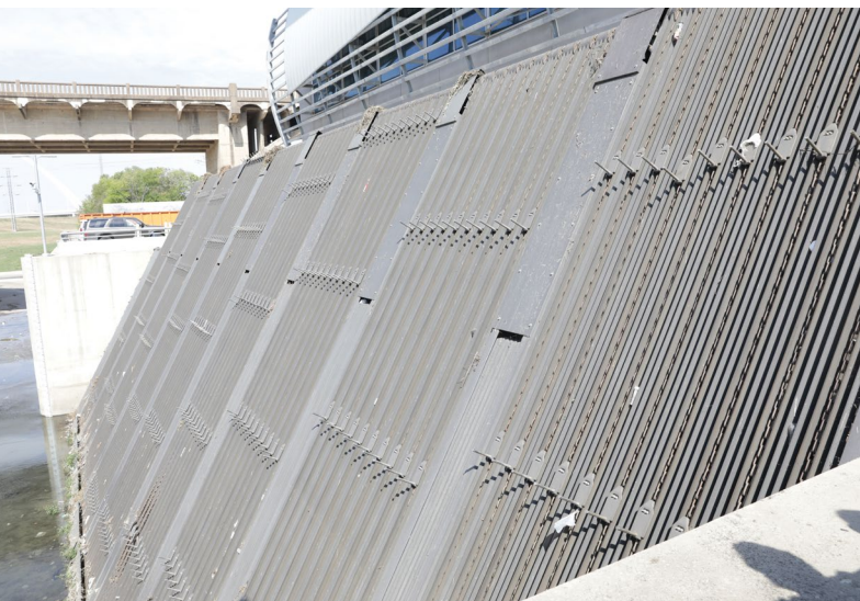
The Able Pump Station was the latest stop on the Engineering and Public Works Roadshow (exterior shown).
